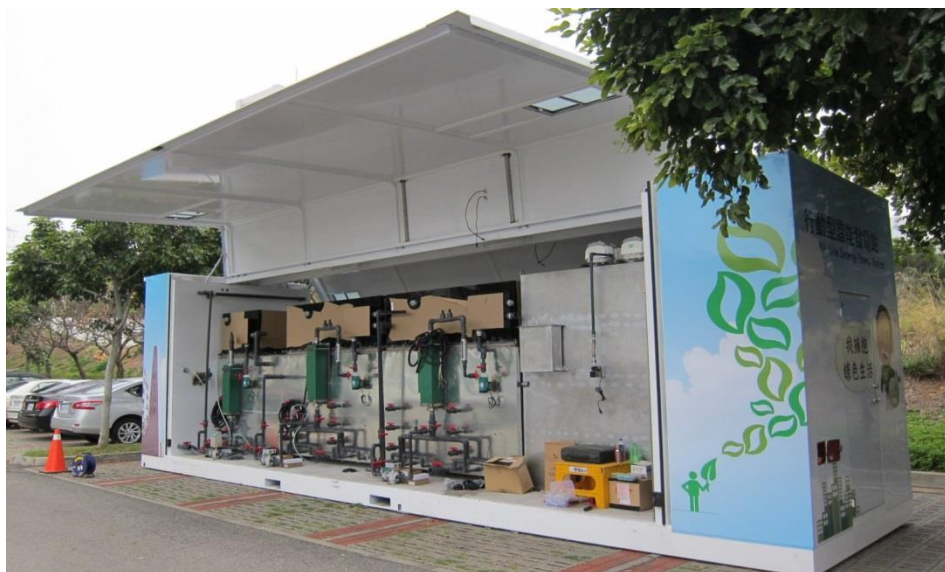
Figure 2. Mobile biogas synergy power pilot plant designed by the Green Energy Development Center, Feng Chia University, Taiwan
