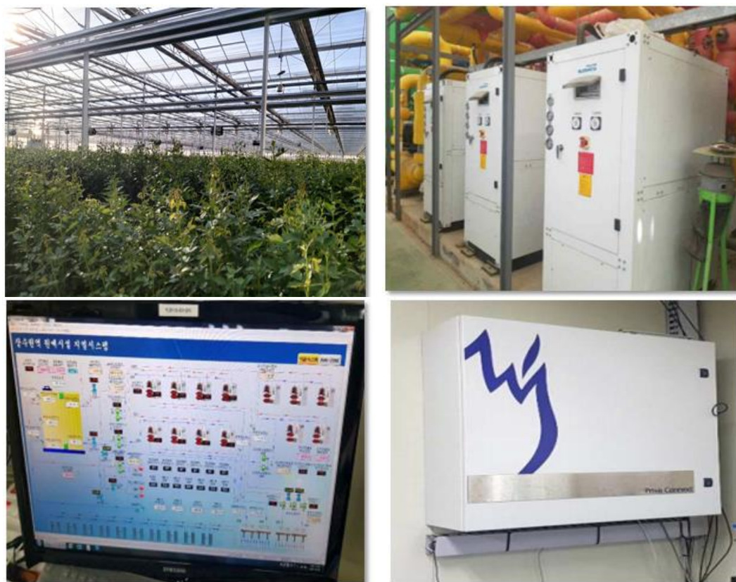
Fig.3. Geothermal heat pump facility of the farm and complex temperature control system
