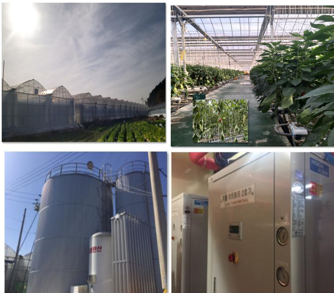
Fig.1. (Above) A view of the farm's geothermal facility, (Below) Heat storage tank and geothermal heat pump facility of the farm
