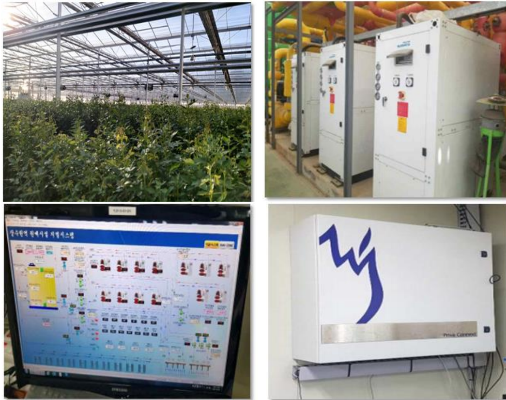
Fig.3. Geothermal heat pump facility of the farm and complex temperature control system
